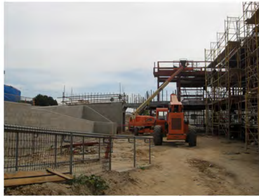
existing ADA ramp on right to remain, new ADA ramps beyond on left, ADA bridge to be added beyond
