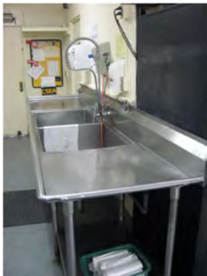
Kitchen equipment to be upgraded during WSM
