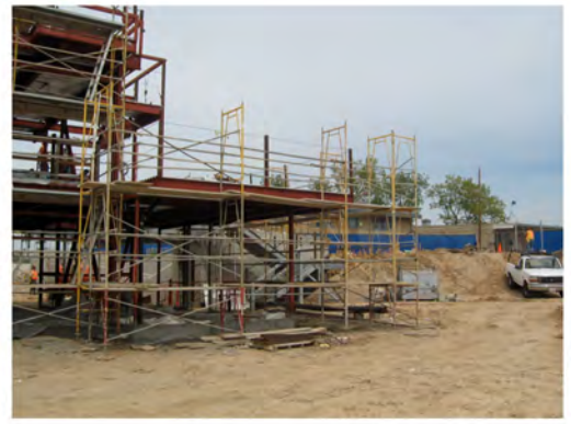
elevator to be in this area, ADA ramp to connect 2nd story to main campus
