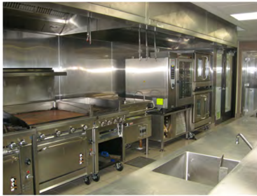
new stoves, ovens & exhaust systems
