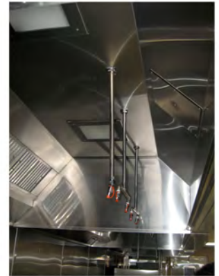
fire suppression systems
