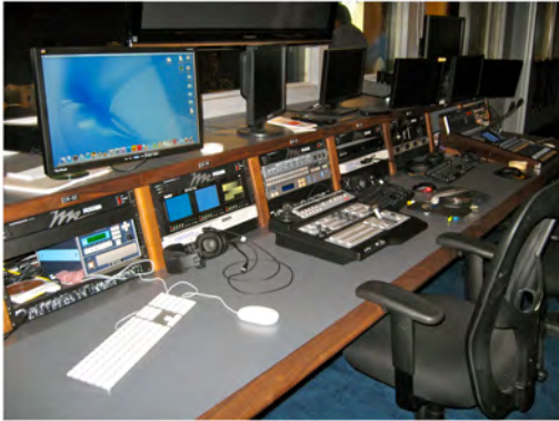
Renovated Multimedia Studio
