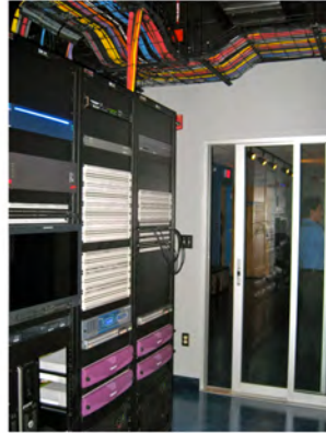
digital media data processing room
