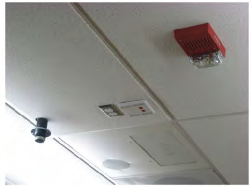
Upgraded fire alarm, lecture amphification (overhead projector provisions, not used by new SmartBoard)
