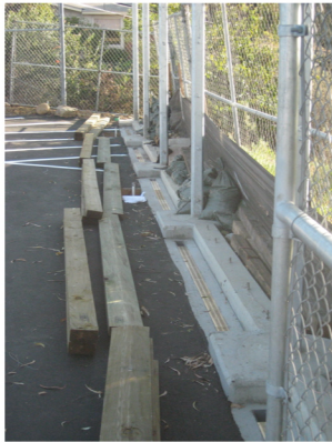
site run-off collection & drainage along West side
