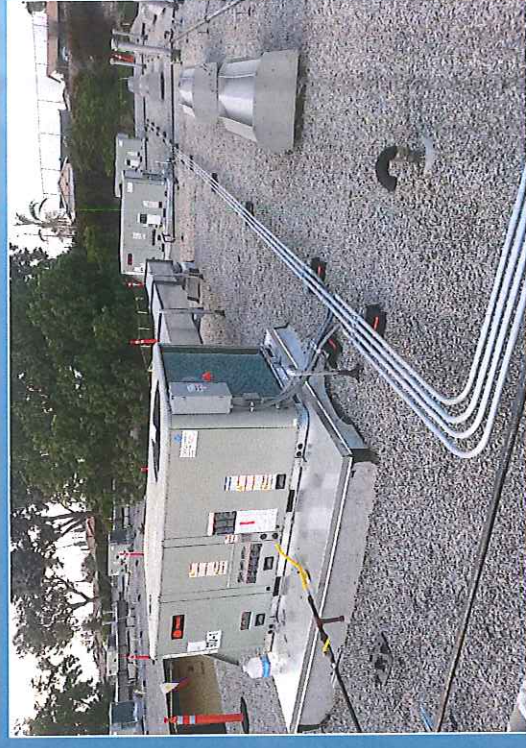
Rooftop-mounted Air Conditioning Equipment At Fulton Elementary
